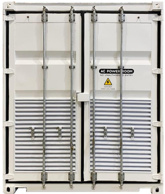
Access point: AC section
